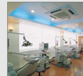
4-way Ceiling Cassette Type
